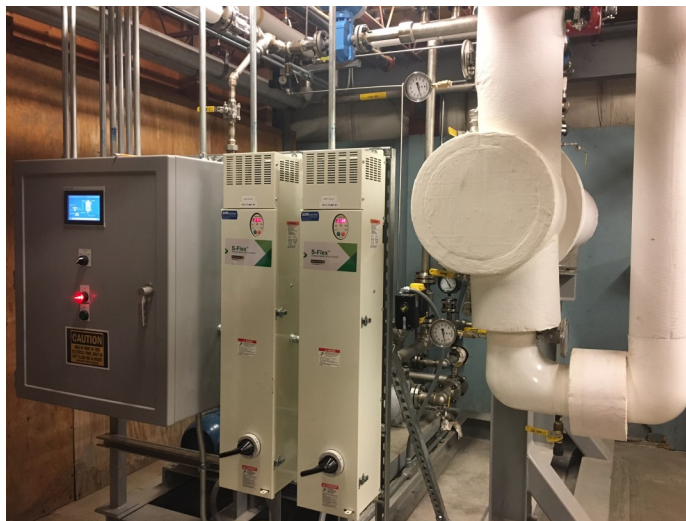
RFO Pump and Heating Skid
